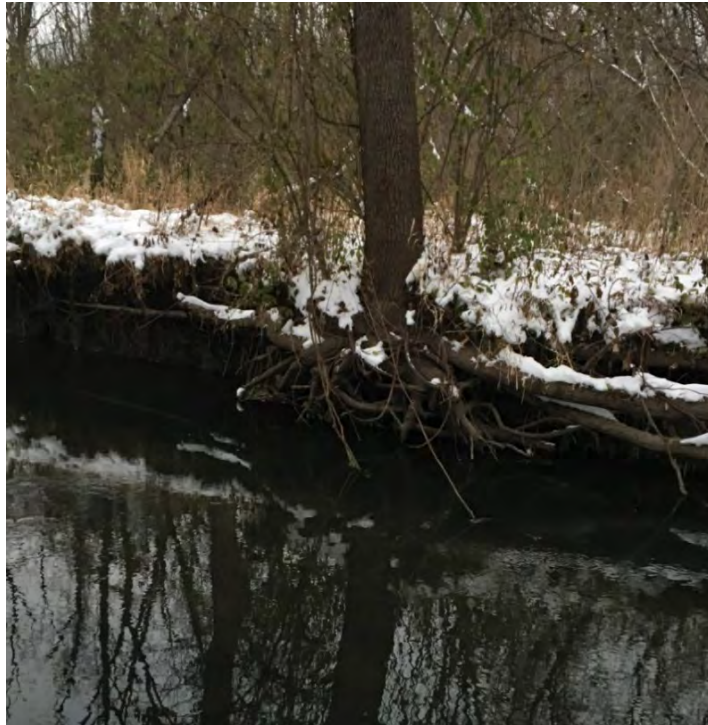
Very severely eroded streambank with tree roots exposed
