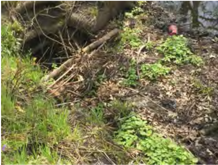
North pond pipe clogged in with mud. Photo credit Lou Ann Johnson, Park-er-Woods Drainage Commissioner
