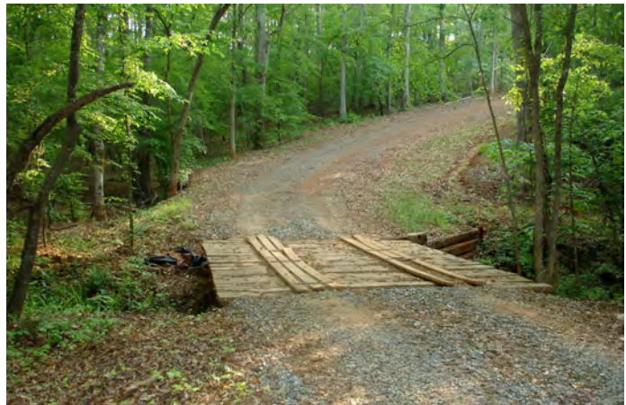
Bridge Crossing (Massachusetts DEP 1997)
