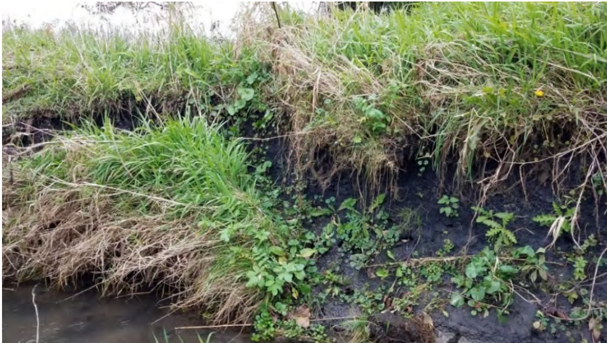
Severely eroded streambank
