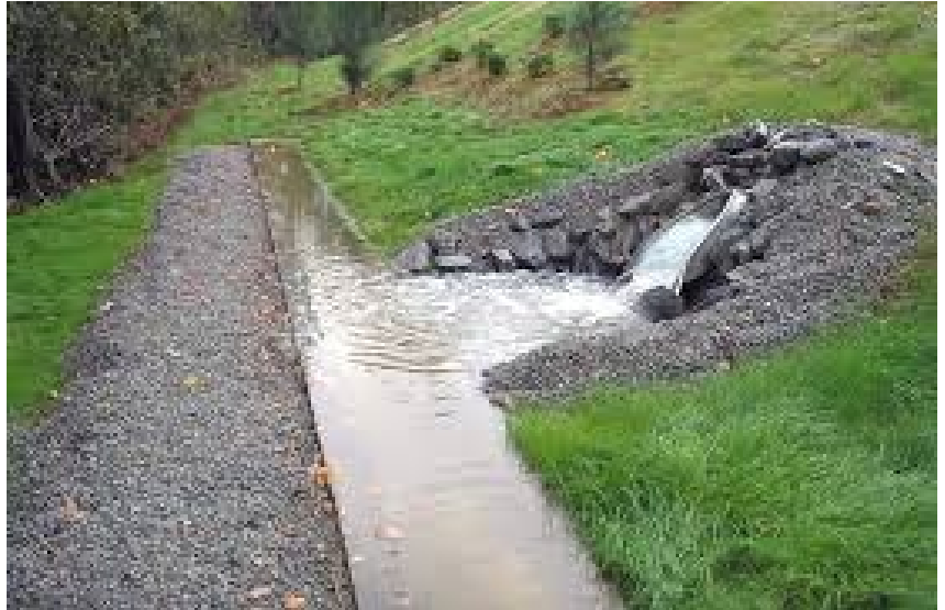
Level Spreader redistributing concentrated runoff from culvert. ( Source : North Carolina Cooperative Extension)
