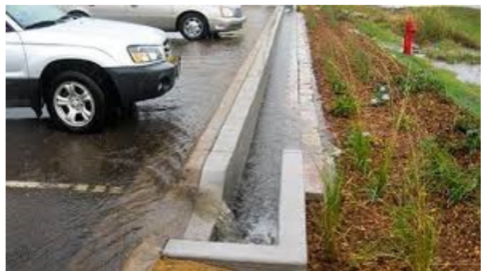
Level Spreader from urban parking lot leading runoff into vegetated buffer strip.
