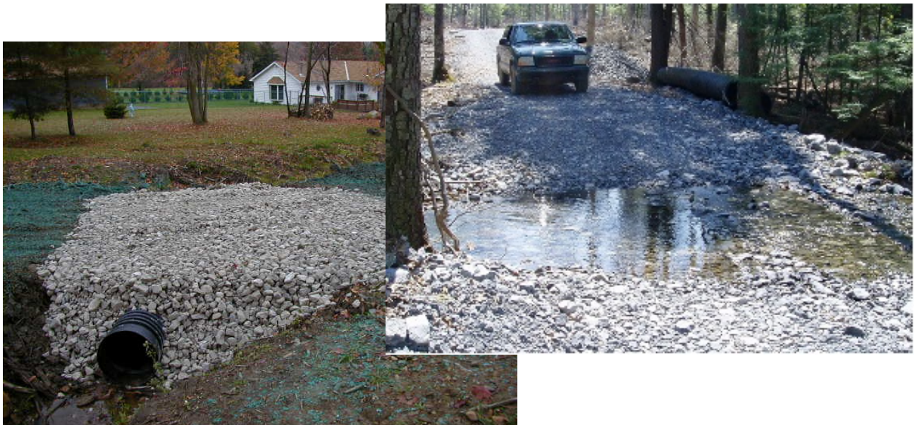
Culvert Crossing (left) and Ford Crossing (right) (Source: Massachusetts Department of Environmental Protection, 1997)
